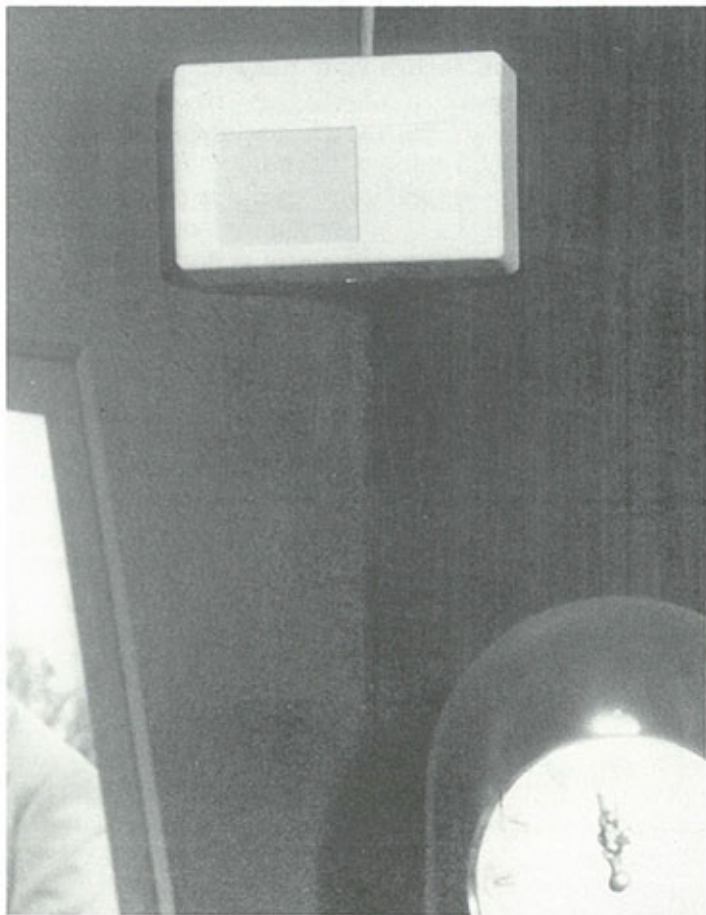
The most common form of space movement detectors, the passive infra-red detector.
